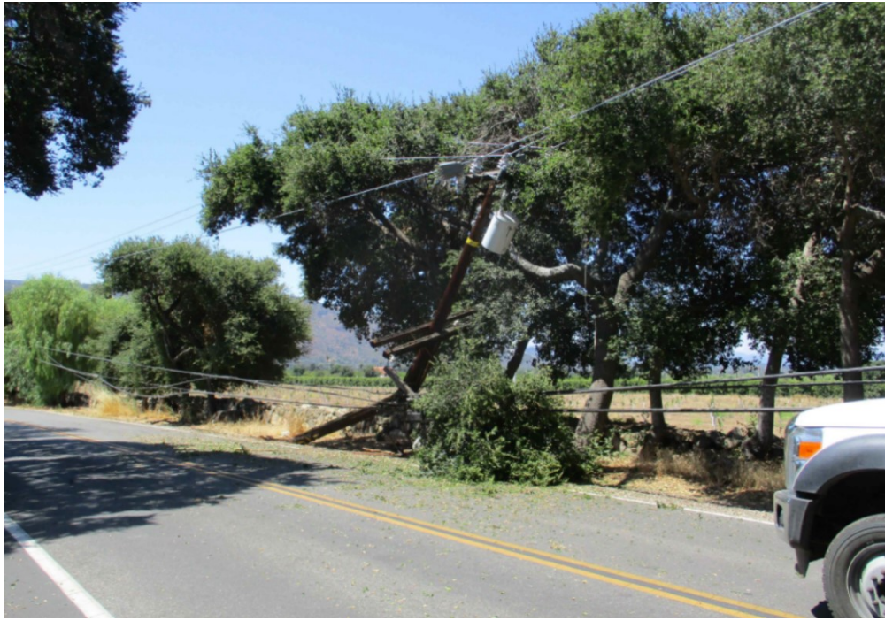
Figure SCE 9.10-5 Covered Conductor Contact with Vegetation After Car-Hit-Pole Ojai, California – July 24, 2020
